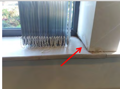
4. Leak Site Below – staining to cills
