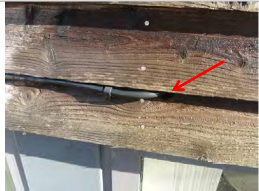
79. Unsealed cable penetration (Recommended Repair) – spray tested – no result
