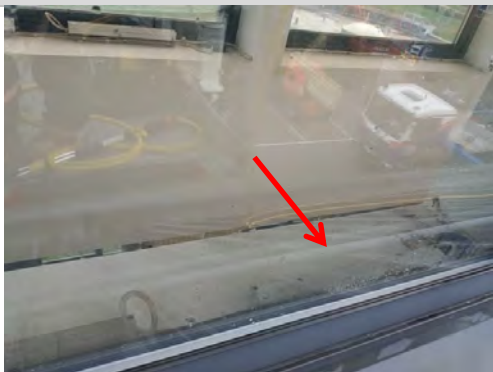
96. Leak Site Below – Leak Duplicated to internal cill
