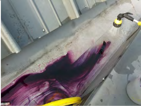
52. Purple dye flood test to defects/gutter waterproofing
