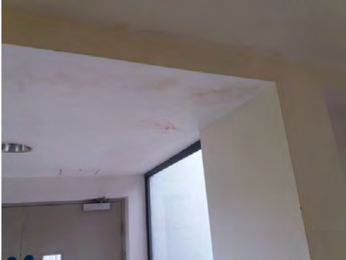
30. Leak Site Below
