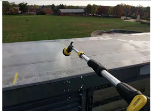
111. Defects sprayed – no result
