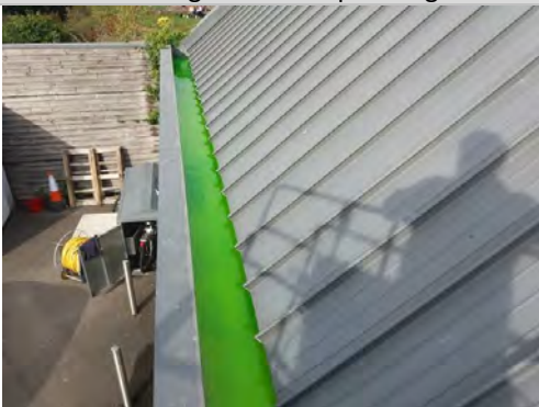
84. Green dye flood test to defect/gutter waterproofing
