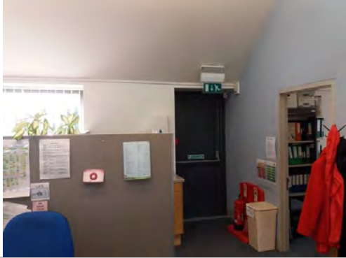
58. Leak Site – fire exit door
