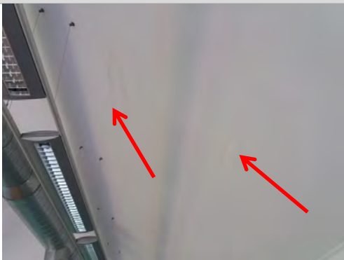
114. Leak Site Below
