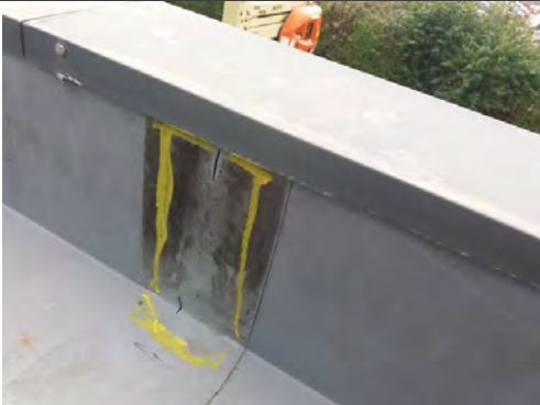
82. Multiple defects (failed butt straps) to box gutter waterproofing
