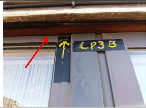
75. Failed/unsealed head of window framework/timber bead (LP3B)
