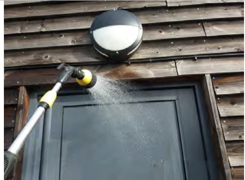
61. Head of door and framework – spray tested
