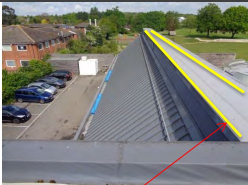
9 Multiple lap defects to roof edge details
