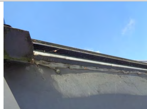
8 Mastic pointing under window. (Poor)
