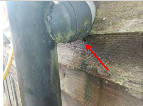
55. Purple dye seeping from the cladding
