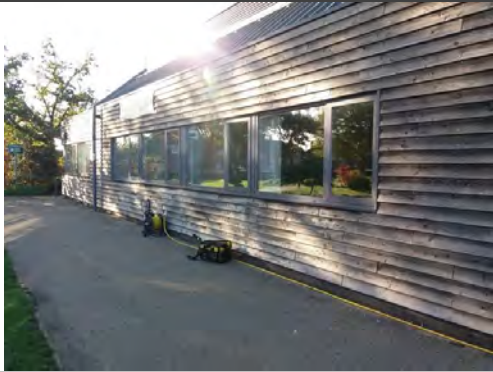
9. Leak Site – external view
