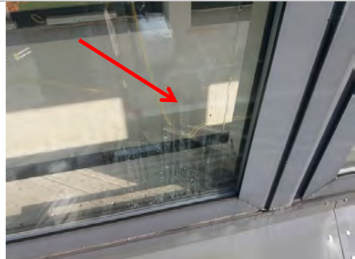
105. Leak Duplicated, tracking down internal glazing
