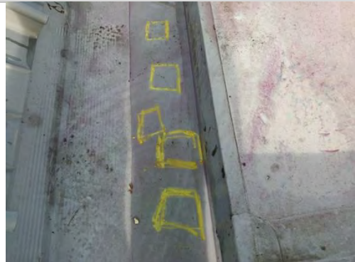
51. Multiple defects/failed butt straps to gutter waterproofing identified
