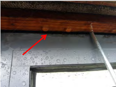
34. Failed/unsealed head of window framework/timber bead (LP2)
