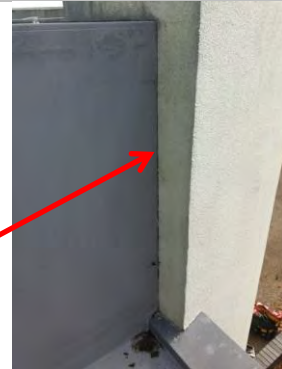
57. Unsealed vertical single-ply joint/abutment to render (Recommended Repair)
