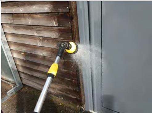
62. Head of door and framework – spray tested
