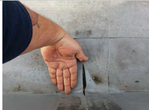
49. Multiple defects/failed butt straps to gutter waterproofing identified
