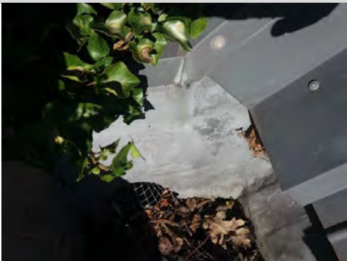
80. Debris blocking gutter, cleared prior to testing
