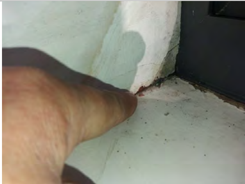
13. Leak Site Below – Leak Duplicated
