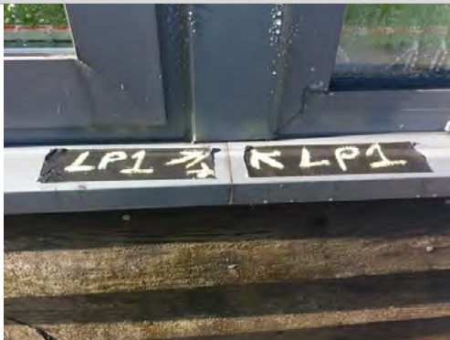
11. 2 Failed/unsealed window cill joints identified (LP1)
