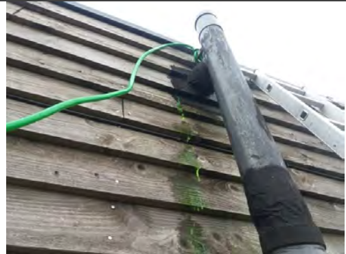
26. Green dye seeping from the cladding
