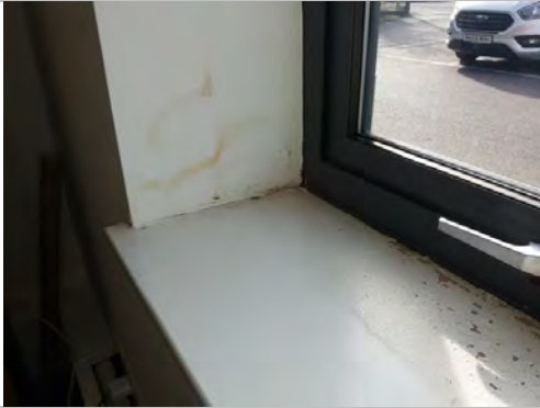
68. Staining to cills/heads of windows
