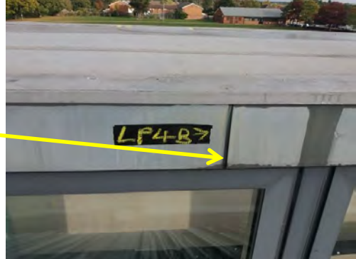
103. Failed/unsealed flashing joint to head of window (LP4B)
