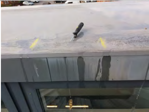
108. Multiple lap defects to flat roof waterproofing identified, above the windows (Recommended Repairs)
