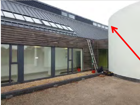
56. Unsealed vertical single-ply joint/abutment to render (Recommended Repair)
