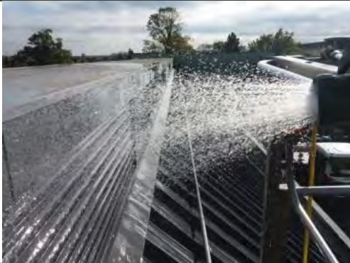
106. Adjacent windows/louvre – spray tested – no result
