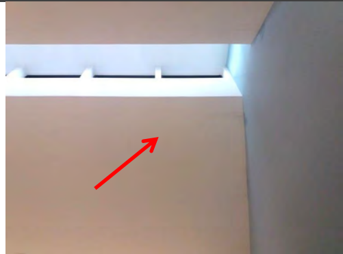
99. Leak Site Below – Leak Duplicated
