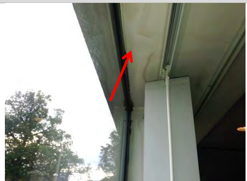
24. Leak Site Below – Leak Duplicated
