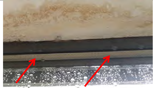
37. Leak Site Below – Leak Duplicated
