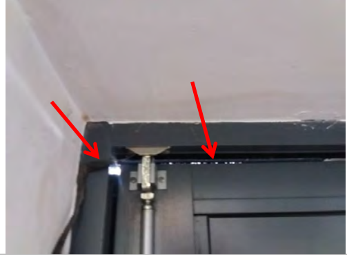
59. Daylight visible to head of door and framework
