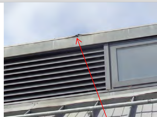
4 Multiple failures of roof trims. (1 example shown)
