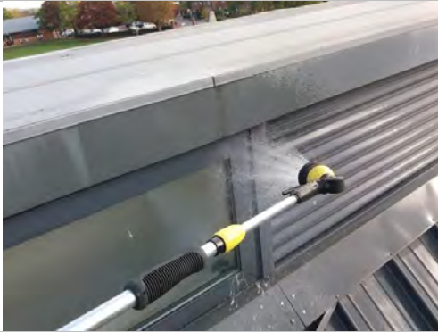
118. Window framework/joints/seals – spray tested – no result
