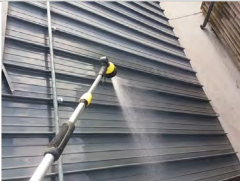
116. Pitched metal roof sheets – spray tested – no result
