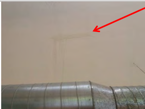
122. Leak Site Below – Leak Duplicated
