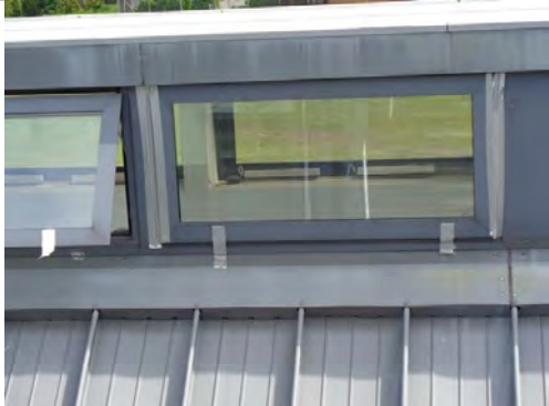
15 Temporary tape repairs to window.
