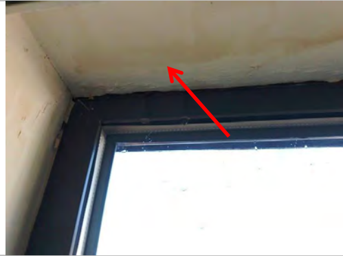
69. Staining to cills/heads of windows
