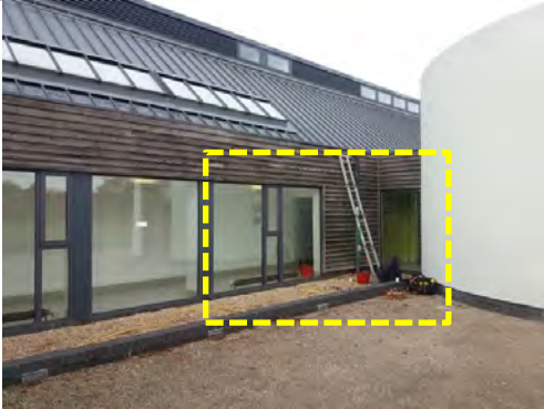
32. Leak Site – external view
