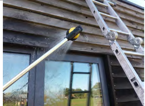
18. Head of window framework/timber bead – spray tested – no result
