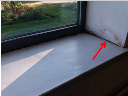
5. Leak Site Below – staining to cills
