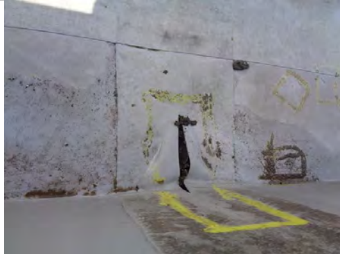
16 Typical of multiple gutter membrane failures
