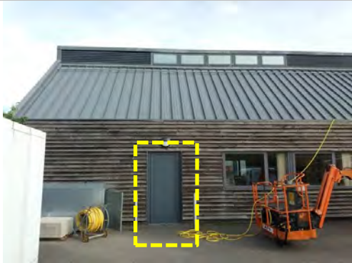
60. Leak Site – external view
