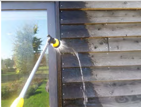
15. Window framework side abutments to cladding – spray tested – no result
