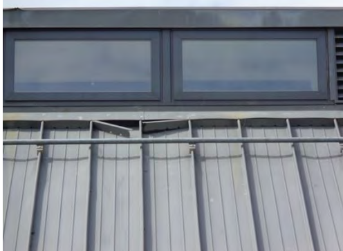
11 Closers slipping in several areas.
