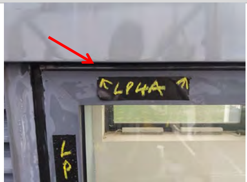
97. Failed unsealed joint to head of window framework (LP4A)
