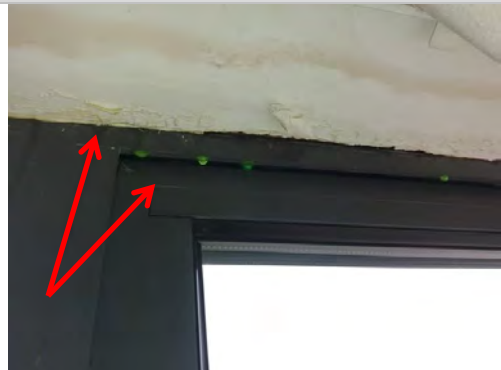
87. Leak Site Below – Leak Duplicated
