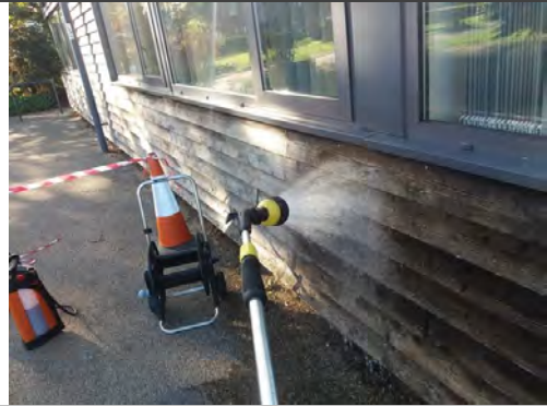
10. Timber cladding, below window cill – spray tested – no result
