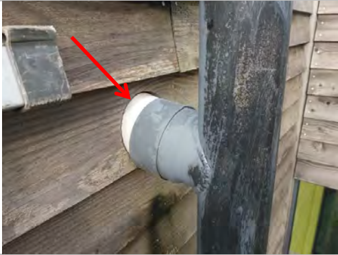
38. Unsealed pipework penetration to cladding (Recommended Repair)
