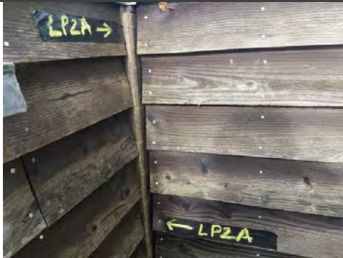
44. Failed/unsealed vertical corner cladding joint (LP2A)
