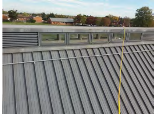
91. Leak Area Above
