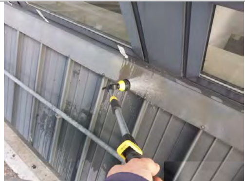
117. Flashing joints/base of windows - spray tested – no result
