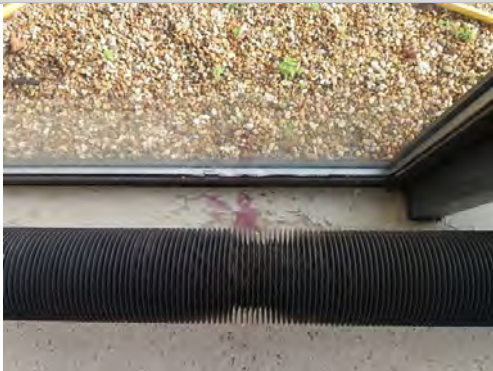
54. Leak Site Below – Leak Duplicated
