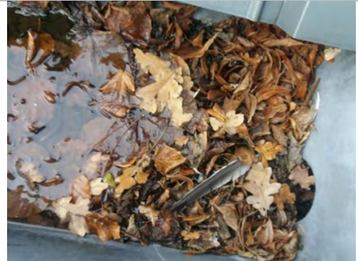
20. High levels of debris cleared from gutter
