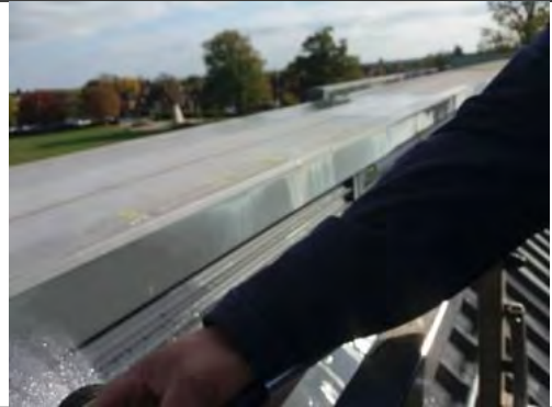
107. Adjacent windows/louvre – spray tested – no result
