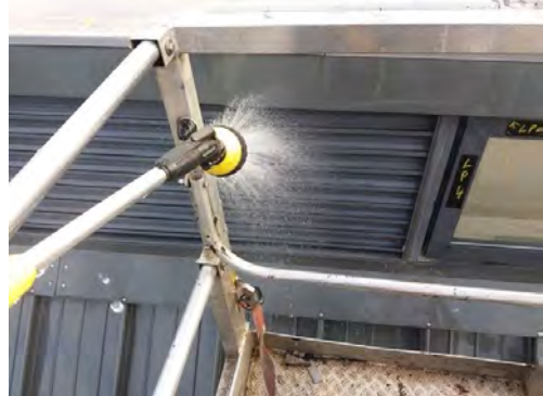
101. Louvre/cill – spray tested – no result
