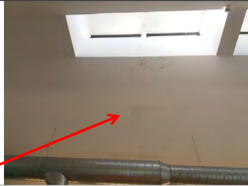
121. Leak Site Below – Leak Duplicated
