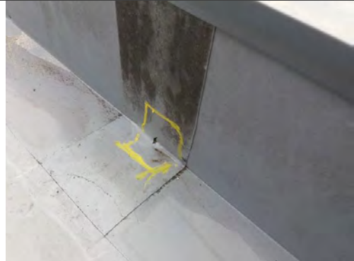
83. Multiple defects (failed butt straps) to box gutter waterproofing
