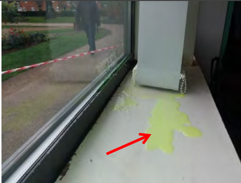
25. Leak Site Below – Leak Duplicated
