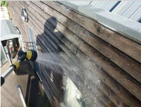
78. Cladding above windows - spray tested – no result
