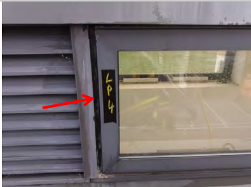
94. Failed/unsealed window framework abutment to louvre (LP4)
