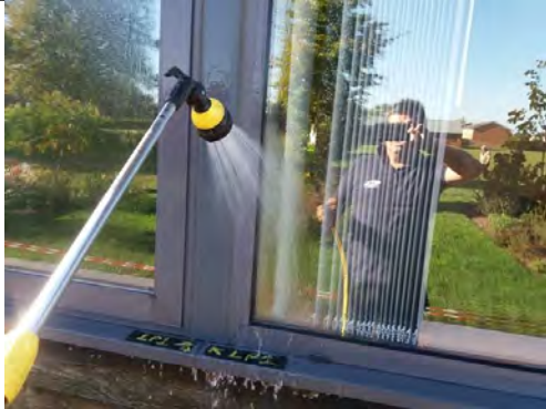
17. Window framework/joints/seals – spray tested – no result
