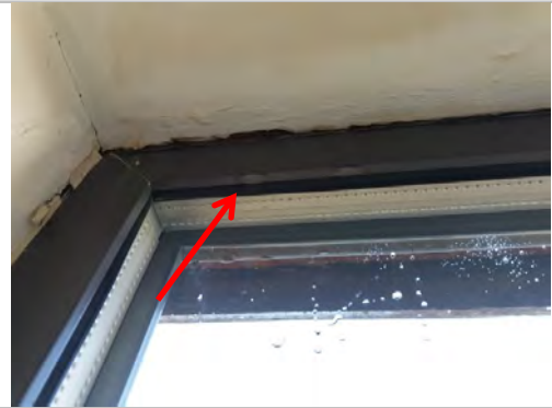
77. Leak Site Below – Leak Duplicated
