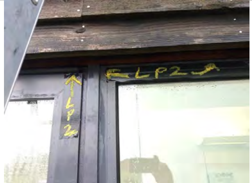
33. Failed/unsealed head of window framework/timber bead (LP2)
