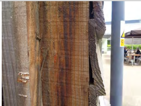
12 Poor finish open ends
