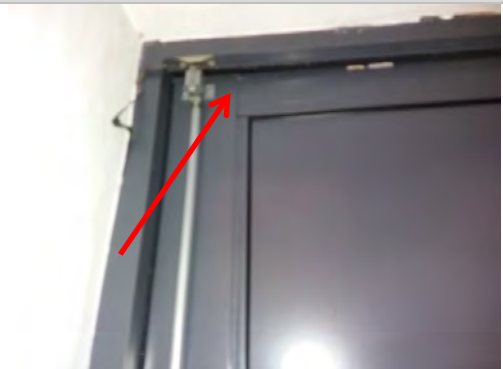
63. Leak Site – Leak Duplicated, tracking down door
