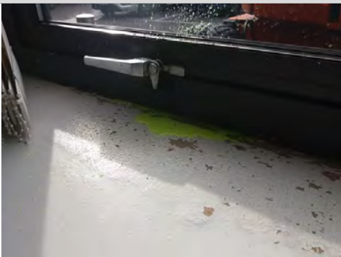
88. Leak Site Below – Leak Duplicated
