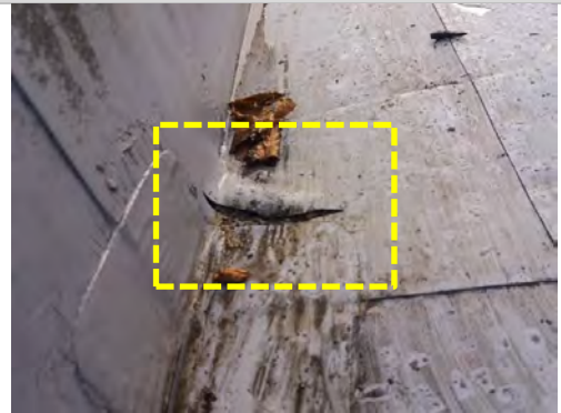
22. Defect (failed butt strap) to box gutter waterproofing (LP1A)
