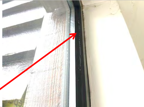
47. Leak Site Below – Leak Duplicated
