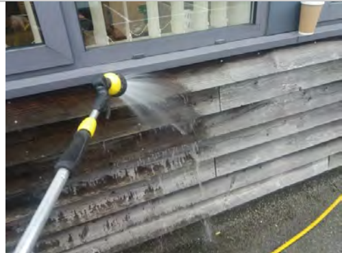
71. Cladding below window cills - spray tested – no result
