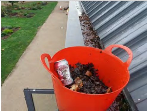
21. High levels of debris cleared from gutter`
