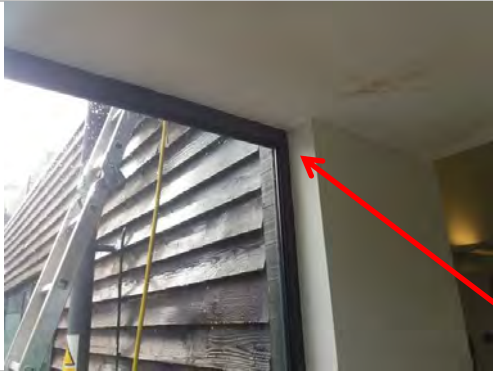
46. Leak Site Below – Leak Duplicated
