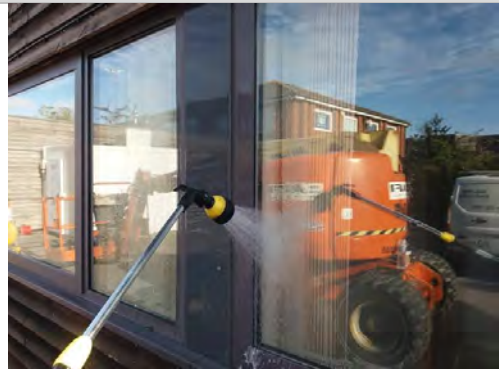
73. Window framework/joints/seals - spray tested – no result
