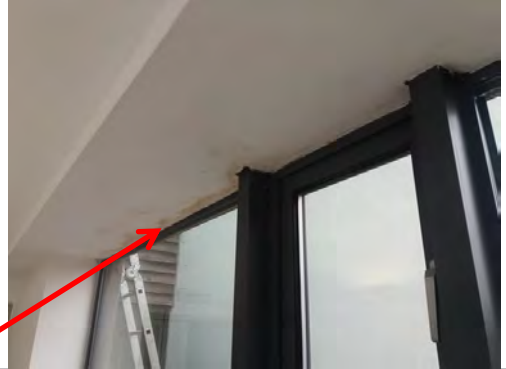
29. Leak Site Below
