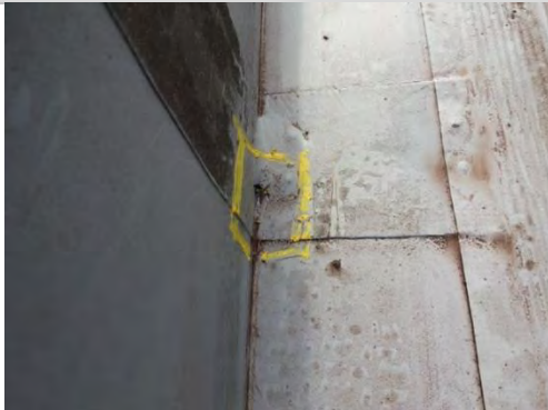
50. Multiple defects/failed butt straps to gutter waterproofing identified
