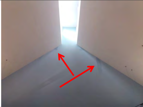
90. Leak Site Below
