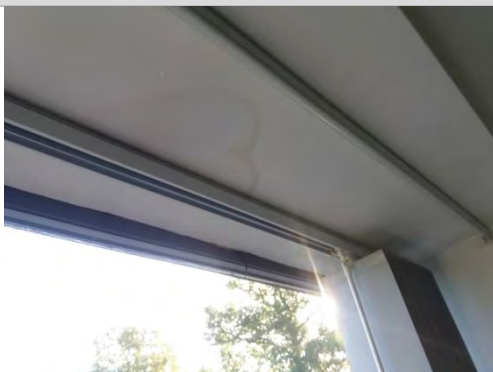
7. Leak Site Below – staining to window heads
