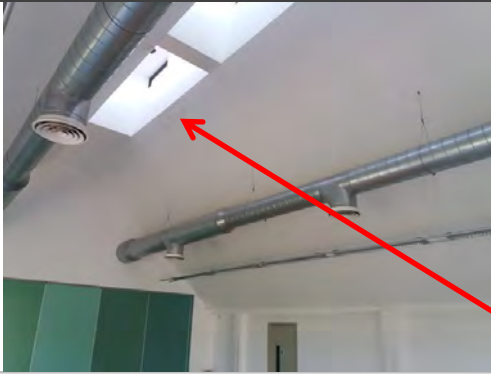
112. Leak Site Below
