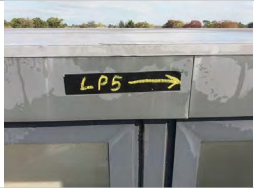
119. Failed/unsealed flashing joint to head of window (LP5)
