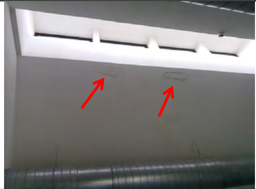
125. Leak Site Below
