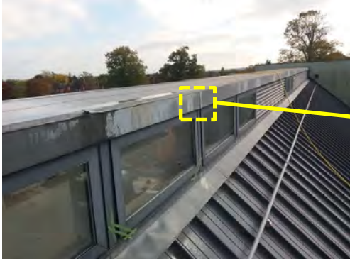
102. Failed/unsealed flashing joint to head of window (LP4B)
