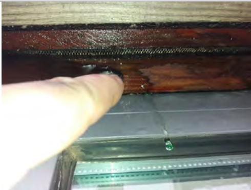
27. Dripping from the external heads of the window frameworks
