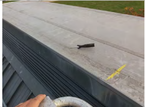
109. Multiple lap defects to flat roof waterproofing identified, above the windows (Recommended Repairs)
