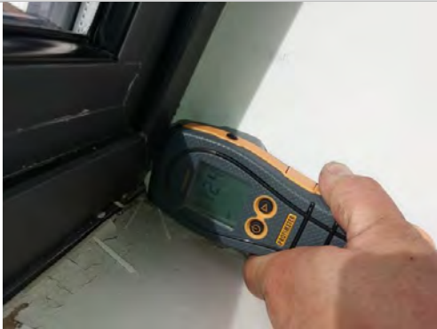
70. Protimeter readings prior to testing gave scale readings of '124 - 141' indicating low levels of dampness
