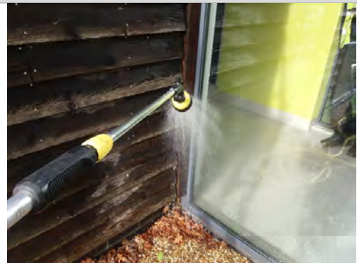
41. Head of window framework and side abutments to cladding - spray tested – no result
