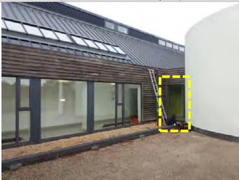
40. Head of window framework and side abutments to cladding - spray tested – no result
