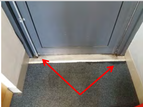
64. Leak Site – Leak Duplicated, tracking down door
