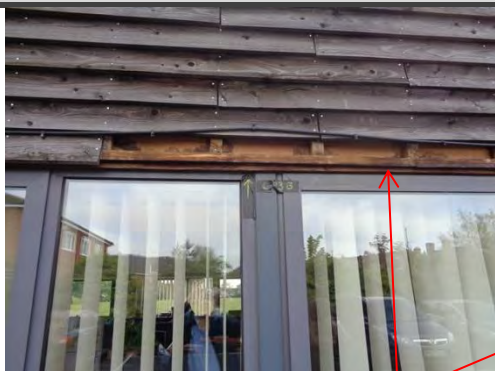
1. Removed cladding, showing no cloaking membrane
